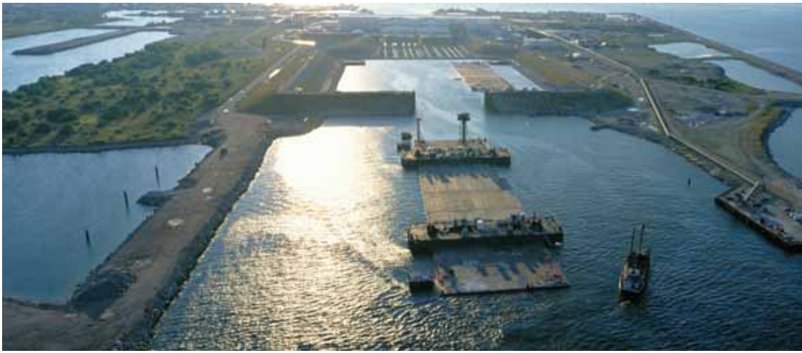
The first tunnel element is towed from the factory at Copenhagen's North Harbour.
